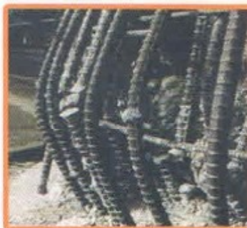
Damage due to insufficient gas pressure welded splices. Longitudinal reinforcement broke at pressure welding portion in Kobe earthquake.
