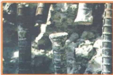
Failed welds at splices of longitudinal reinforcement in a column supporting the Hanshin Expressway (at the 500-meter-long failed section). These gas fusion welds are 1960s technology and are not common today in the United States.
