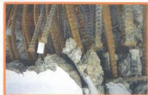
A fairly common feature of bridge column failure was the popping of gas pressure welded splices, which represent fairly common Japanese practice. These splices failed frequently in older buildings, and occasionally in new construction.
