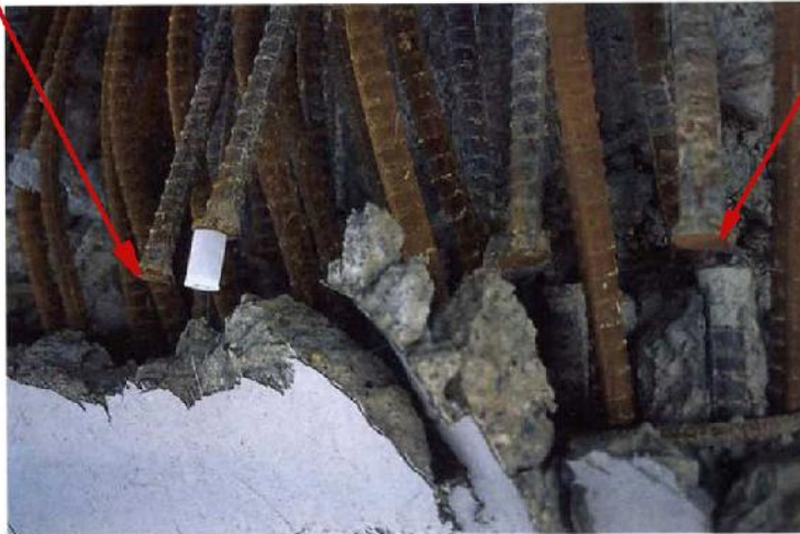
Fig. 6. Failure of "gas-pressure welded" splices in a bridge pier.
